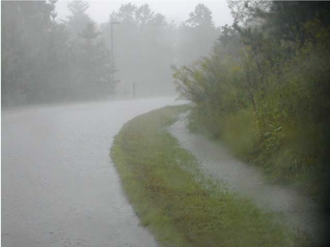
Figure 13: Turf Reinforced Swale conveying runoff.
