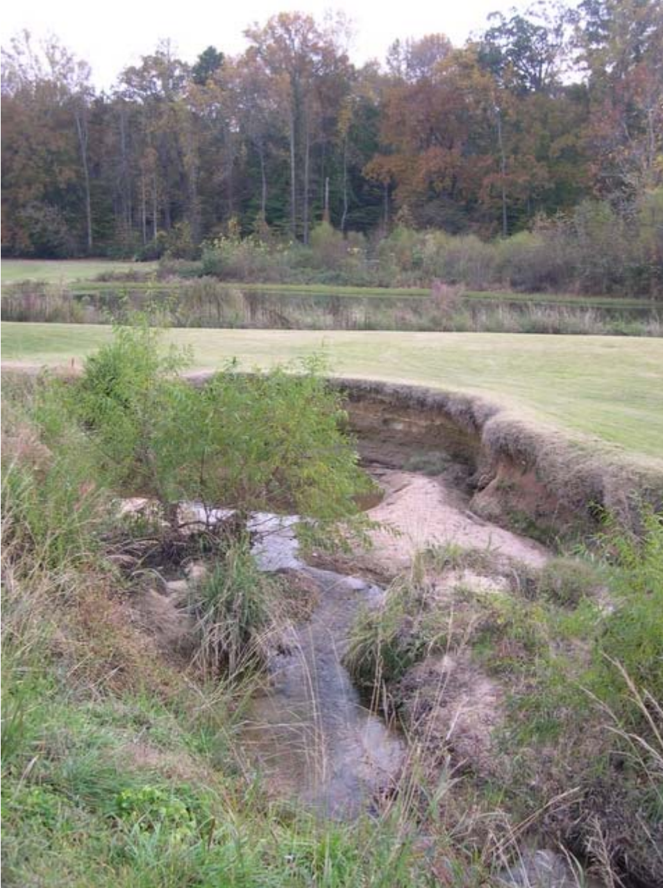
Figure 8: Incised channel without floodplain access
